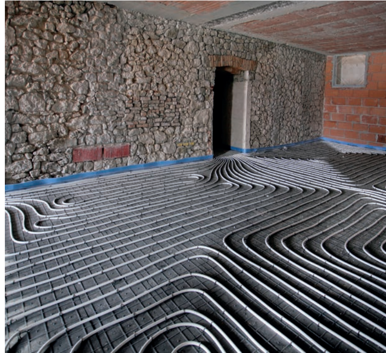
Castle, Italy ▲ Underfloor heating and cooling
