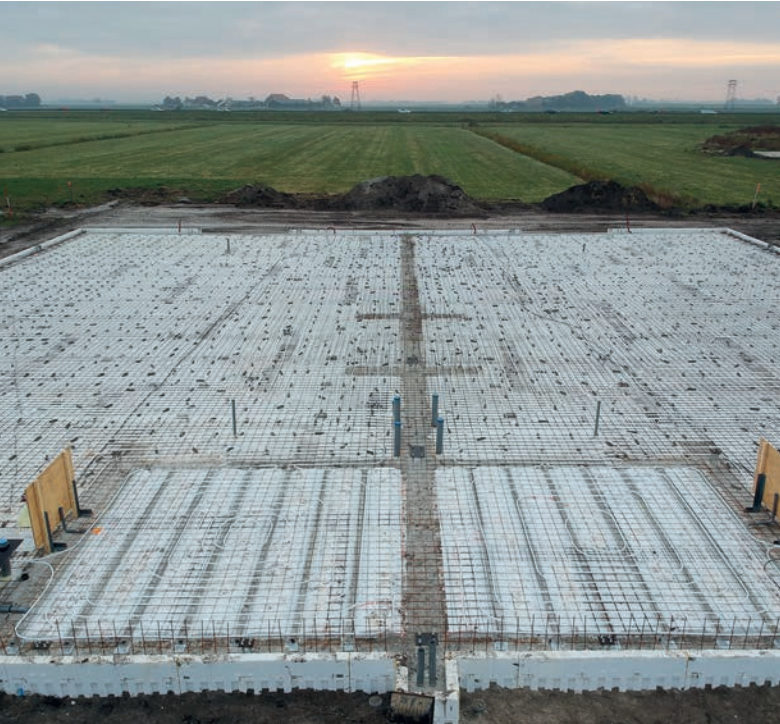
▲ Project Lemmer, Friesland, The Netherlands Underfloor heating
