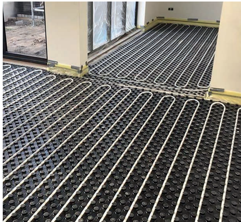
Breda, The Netherlands ▲ Underfloor heating
