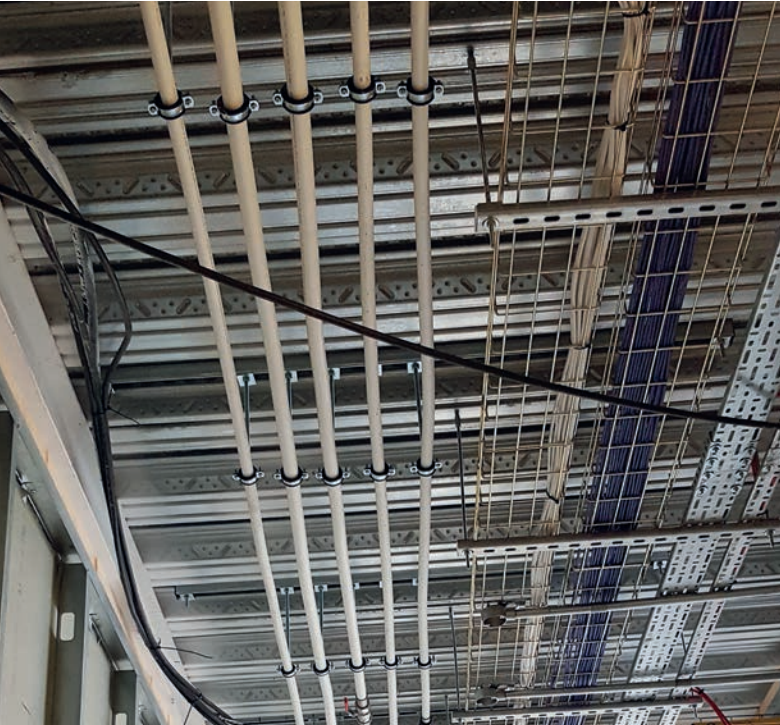
▲ Chichester University, UK Heating and sanitary
