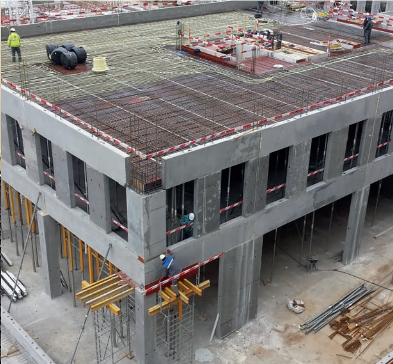
▲ Post X, Antwerp, Belgium Concrete core activation
