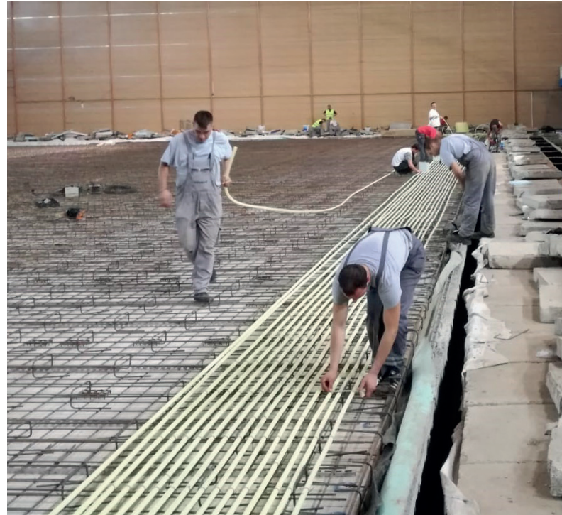
▲ Rink Stadium, Zagreb, Croatia Cooling system for indoor ice skating ring
