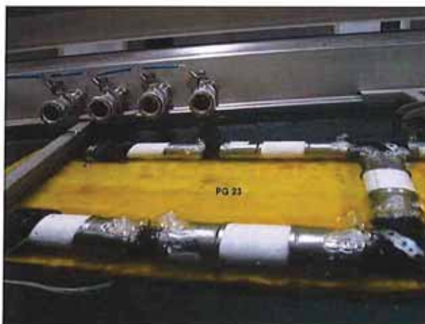
Figure 1: Clear leakage while tested with air
